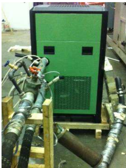
Photo #7 Test unit set-up
