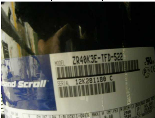
Photo #3 Compressor nameplate
